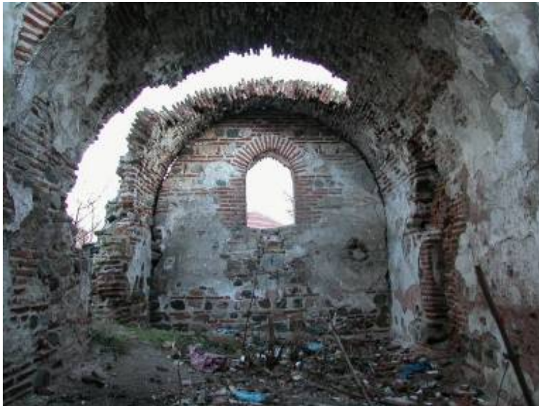
Interior. The sanctuary. Note the partially collapsed state of the barrel-vault and the buckling of what remains of the left-hand side of the vault at its juncture with the mihrab wall.
