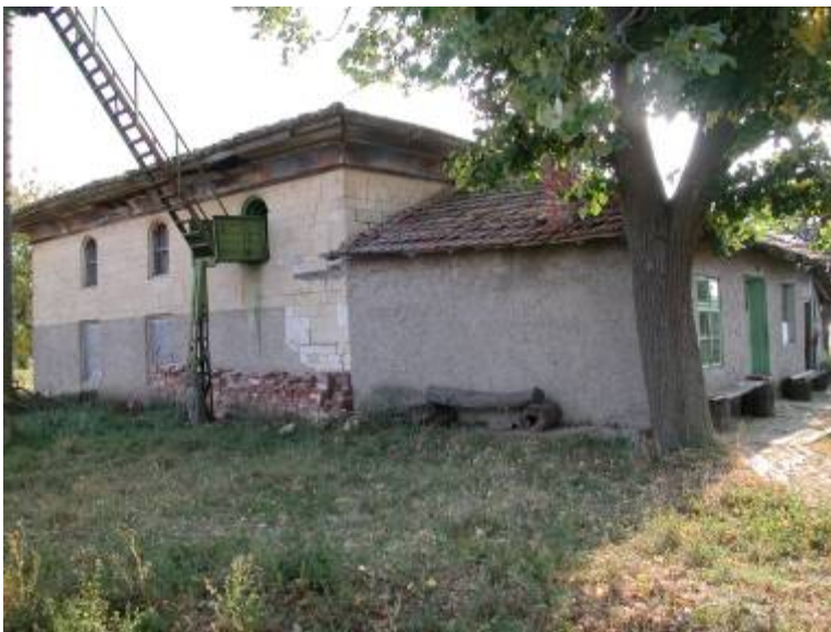
Oblique view from left. Note bricked-in portico, improvised access to minaret, cracks and buckling at left front corner, and laying of brick in an attempt to shore up wall.
