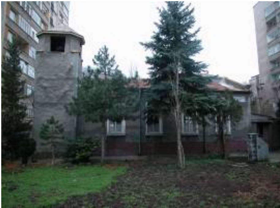
Lateral view from ul. Dobrudja. Despite signs of dampness on stucco walls, roof tiles show evidence of recent repair.
