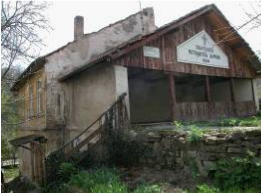
First story entrance and façade of building. Note signs of dampness.
