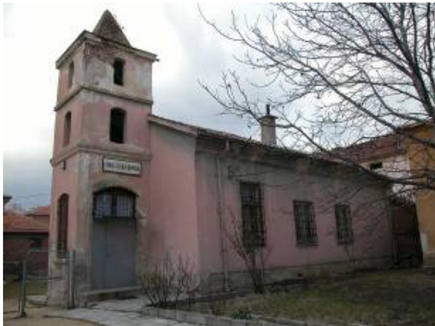
Oblique view. The grey door is a late addition; vestibule under bell tower was formerly open on the sides. Note damage to bell tower.
