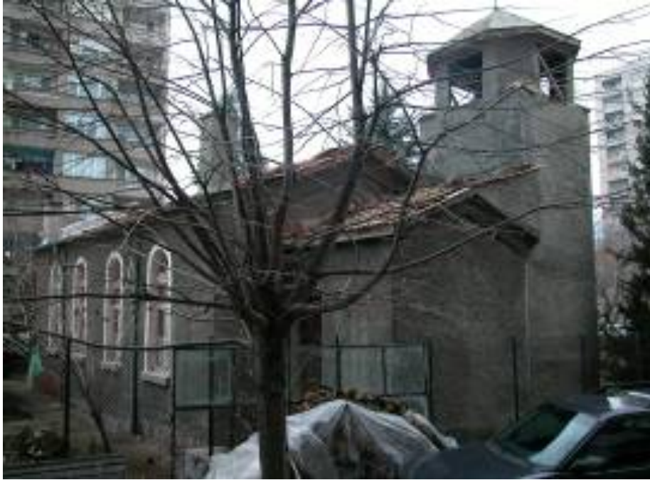
Oblique view from side street towards entranceway. Note walled-in portico and awkwardly placed and executed bell tower, quite possibly a later addition. Exposed brick footing suggests that external walls are of brick.
