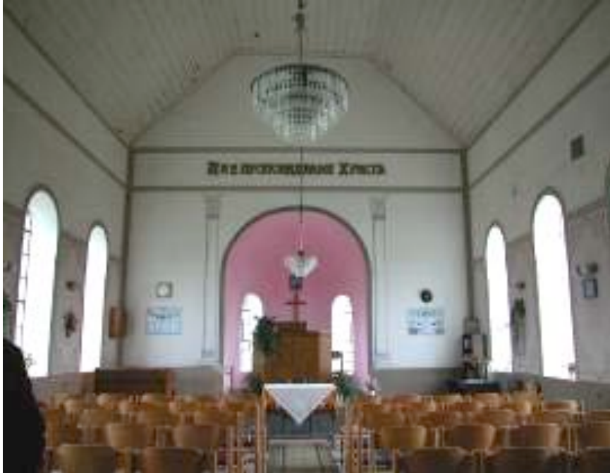
Interior towards altar and apse. Note signs of rot in wood ceiling, especially at juncture with altar-end wall.
