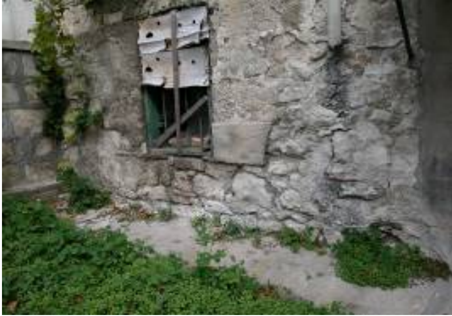
Lower left of façade indicating condition of the exterior walls.
